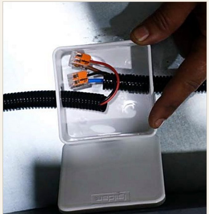
7B · SLEEVED CABLES MEETING THE WAGOS INSIDE THE JUNCTION BOX
